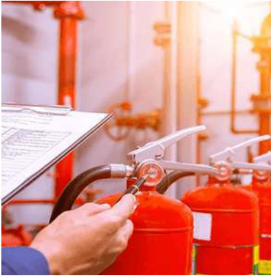
FIRE ALARM & FIRE FIGHTING- AMC SERVICES
